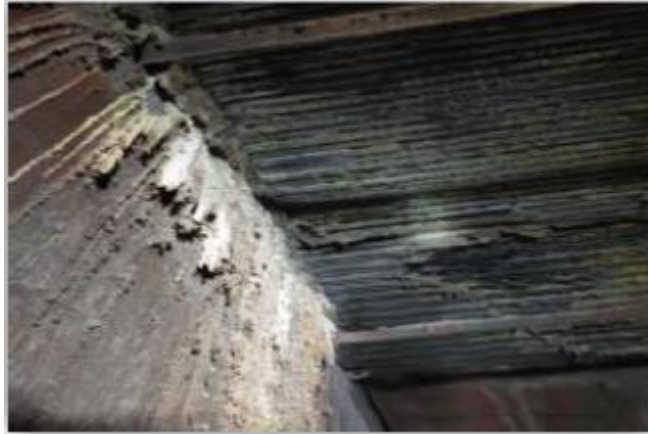
ABS sticks to and clog on the pipes due to polymer deNOx agent
