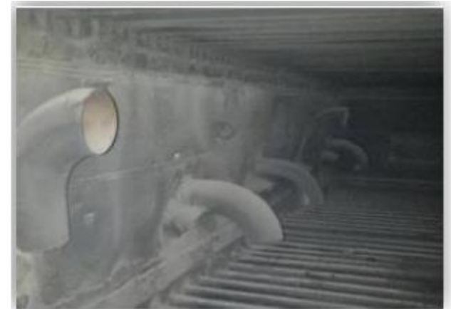
Clean gas duct. The efficiency of heat exchanger is increased.
