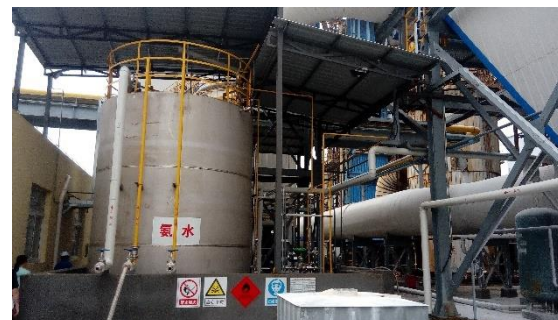
Ammonia Storage Tank
