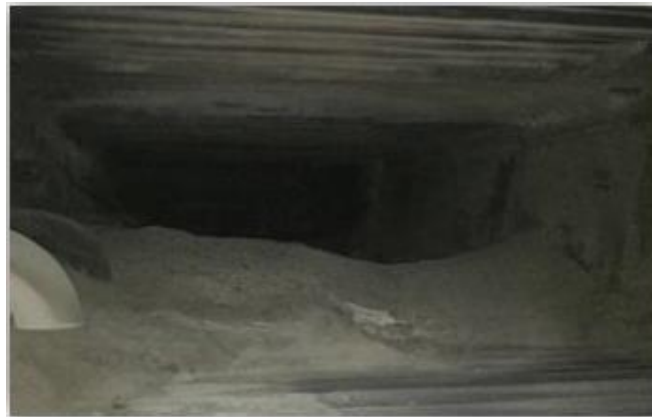
Gas duct clogged by ABS and dust
