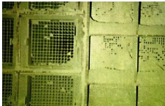
Dust Clogging and wear-out of catalyst
